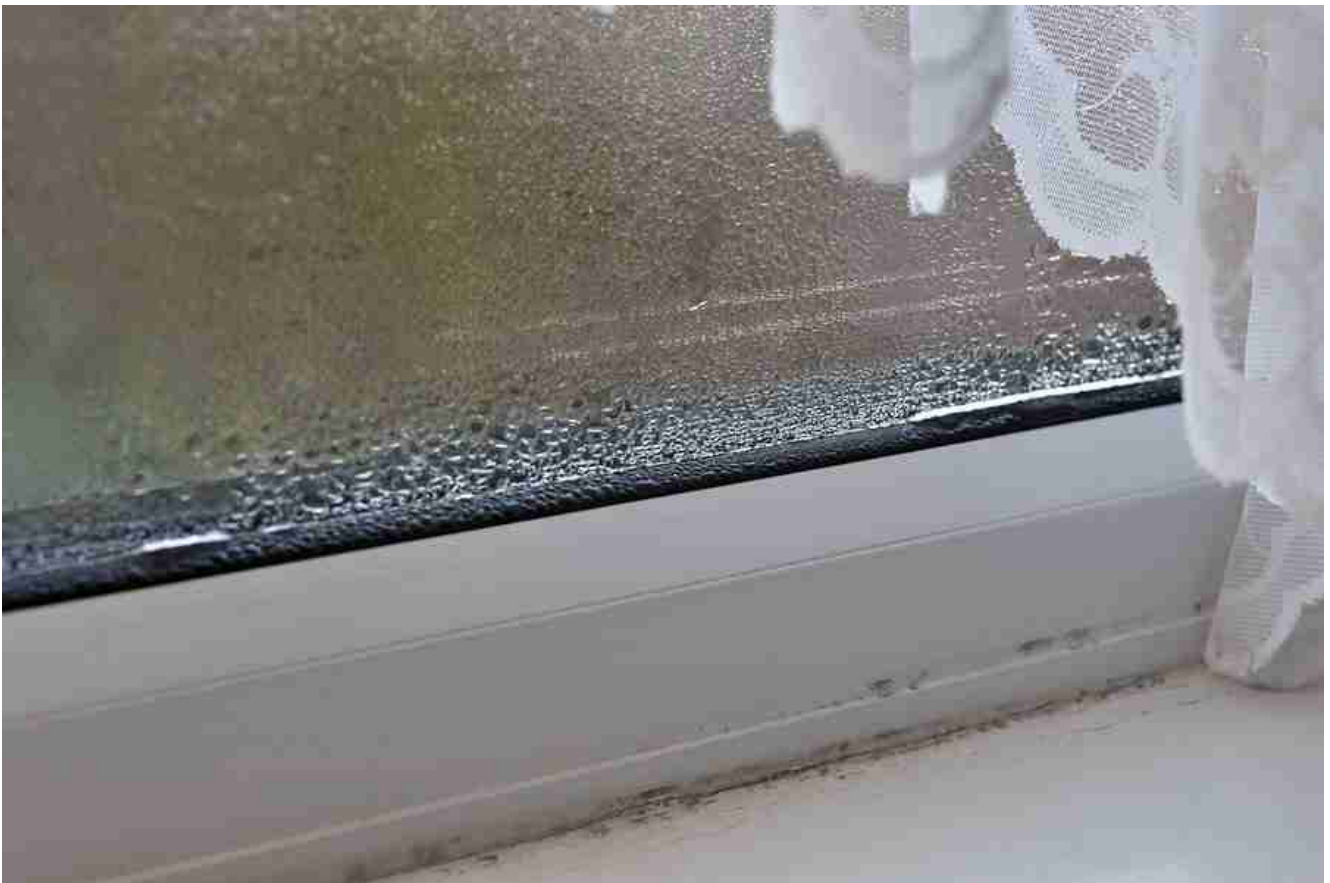
Condensation on the inside of a double glazed window without argon gas filled.
